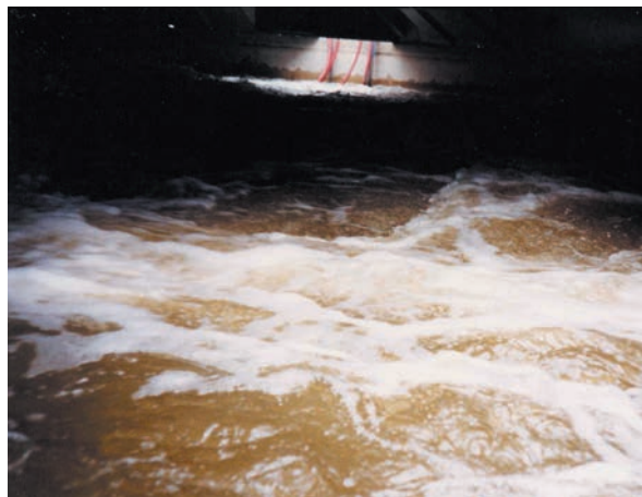
Submersible AirJets in leachate tank
