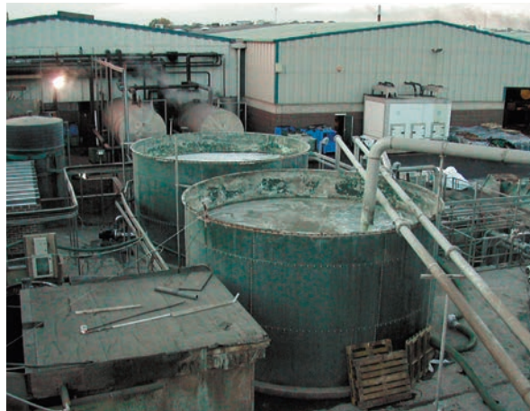
Dry-installed AirJet in tannery effluent aeration tank
