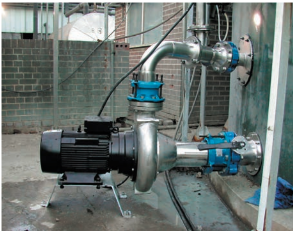
Dry-installed AirJet in tannery effluent aeration tank
