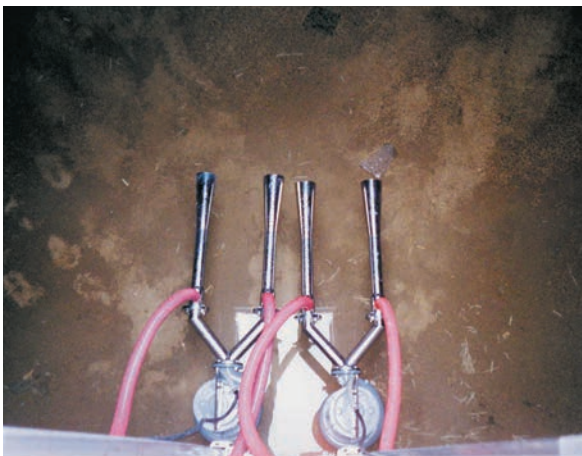
Submersible AirJets in leachate tank
